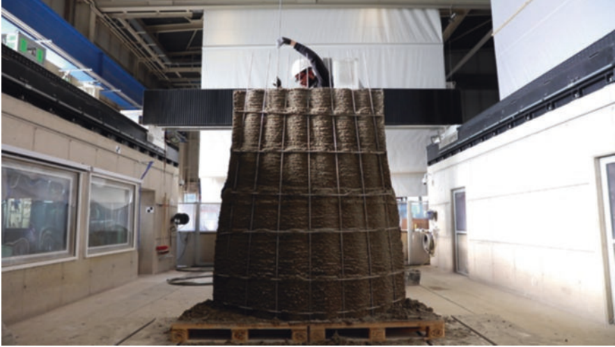
Fig. 3 Threading unbent vertical reinforcement into the shotcrete core structure. (Image courtesy Norman Hack)
